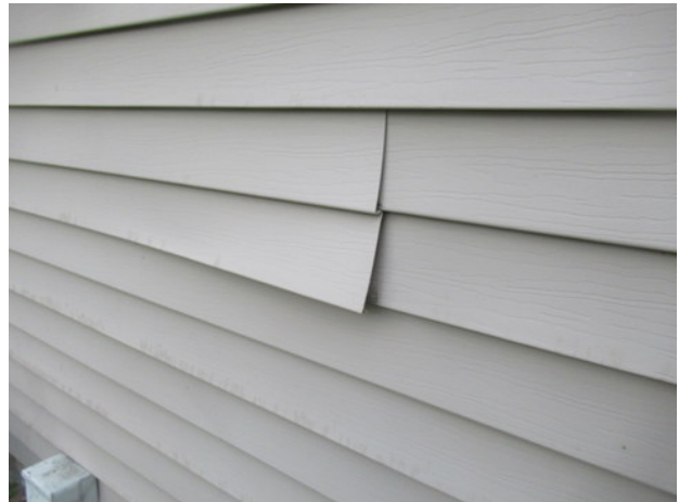
Loose siding and deterioration at vinyl siding of Unit 1304
