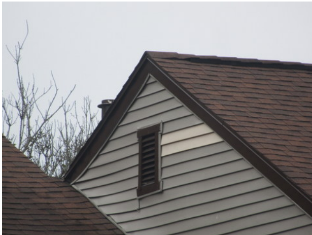
Previous partial siding replacement, warping and deterioration at vinyl siding of Unit 1452
