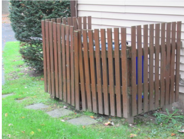
Leaning fence section and deterioration at wood refuse area fences near Unit 251
