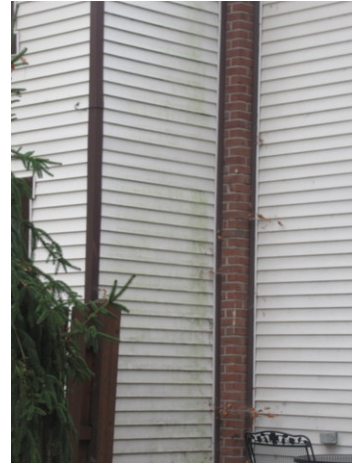
Organic stains and deterioration at vinyl siding of Unit 101
