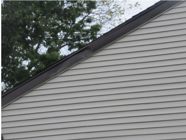
Damage and deterioration at fascia cladding of Unit 1756
