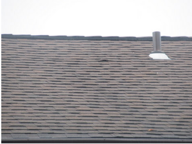
Shingle lift and deterioration at asphalt shingle roof of Unit 554
