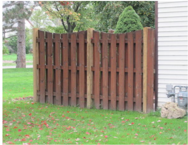
Previous fence post replacement and deterioration at wood privacy fence near Unit 156
