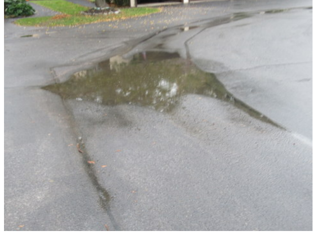
Longitudinal cracks, previous crack and patch repairs, standing water and deterioration at asphalt pavement near Unit 452
