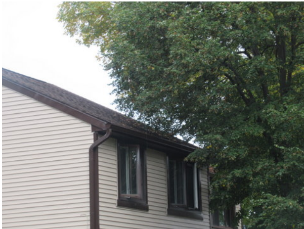
Overhanging and encroaching tree branches, and deterioration at asphalt shingle roof of Unit 603
