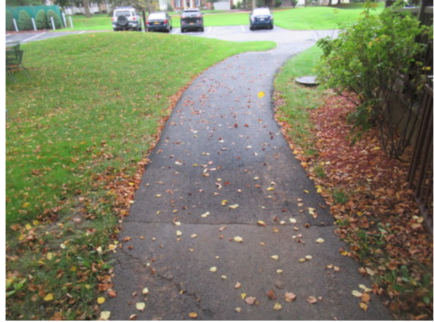
Previous patch repair at asphalt walking path near Unit 603
