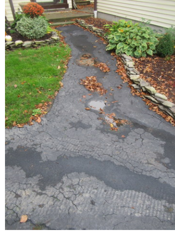
Spider cracks, standing water and deterioration at asphalt pavement near Unit 1253
