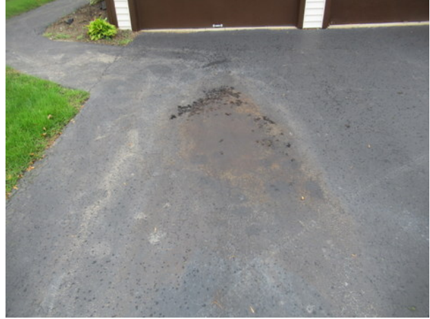
Vehicle fluid stains and deterioration at asphalt pavement near Unit 704
