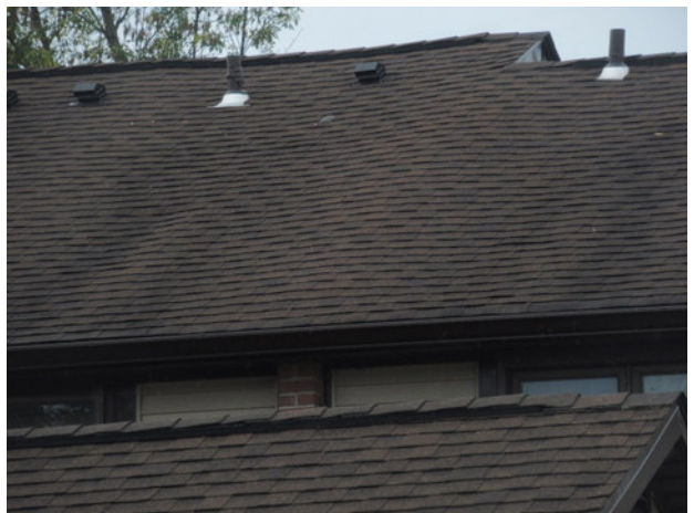
Shingle lift, stains and deterioration at asphalt shingle roof of Unit 551
