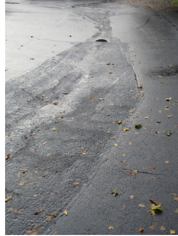
Longitudinal cracks, previous patch repairs, standing water and deterioration at asphalt pavement near Unit 1302
