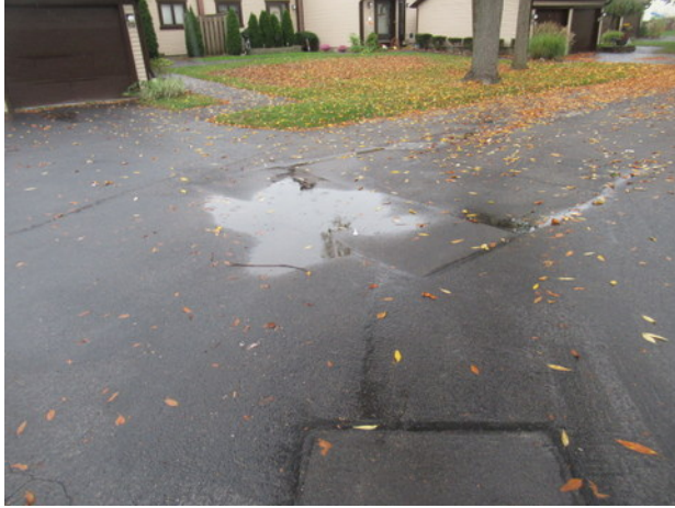
Lateral and longitudinal cracks, previous crack and patch repairs, standing water and deterioration at asphalt pavement near Unit 557
