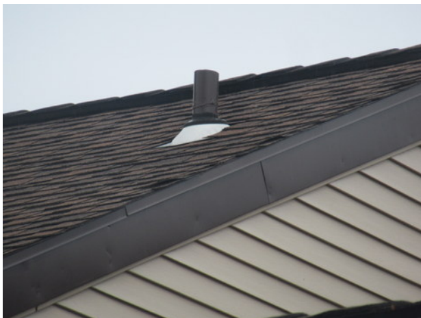
Shingle lift and deterioration at asphalt shingle roof of Unit 356
