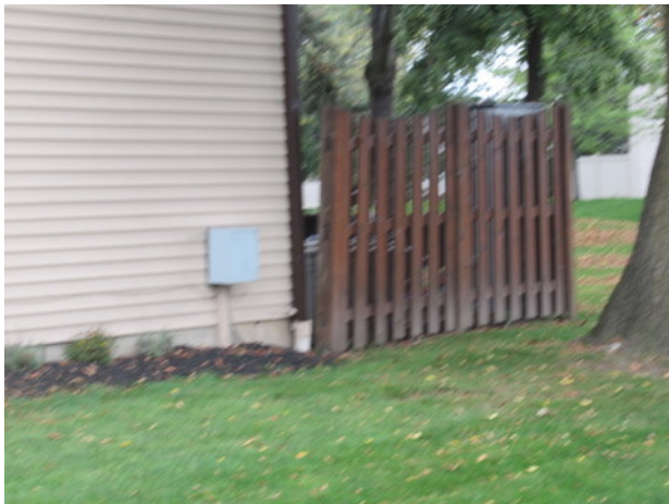
Leaning fence section and deterioration at wood privacy fence near Unit 1408
