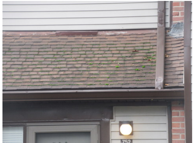
Organic growth and deterioration at asphalt shingle roof of Unit 752
