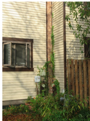
Vegetation overgrowth and deterioration at vinyl siding of Unit 208
