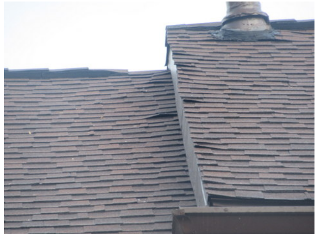
Shingle lift and deterioration at asphalt shingle roof of Unit 907
