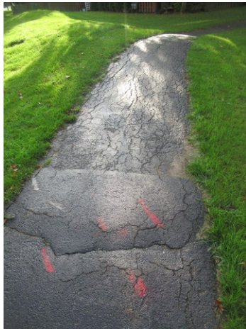
Spider, edge and alligator cracks, previous patch repairs and deterioration at asphalt walking path near Unit 1208
