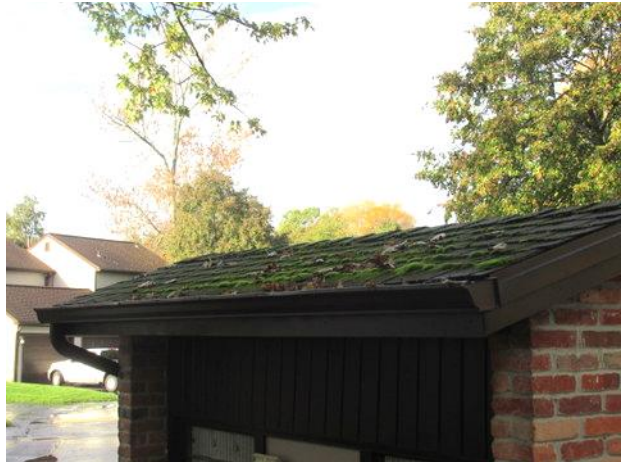
Organic growth and deterioration at asphalt shingle roof of mailbox shelter near Unit 1056
