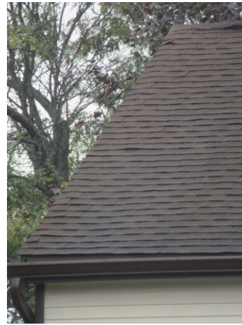
Shingle lift and deterioration at asphalt shingle roof of Unit 301
