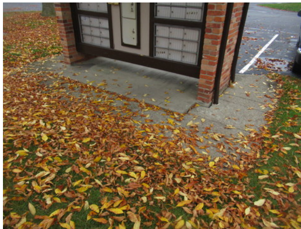
Cracks and deterioration at concrete pad of mailbox shelter near Unit 1454
