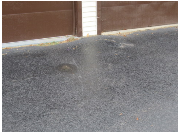
Minor settlement and deterioration at interface of asphalt pavement/garage threshold near Unit 455
