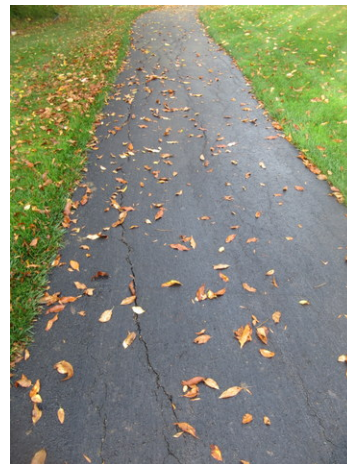
Longitudinal, edge and alligator cracks, and deterioration at asphalt walking path near Unit 706
