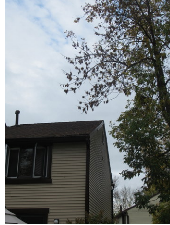
Overhanging and encroaching tree branches, and deterioration at asphalt shingle roof of Unit 1556
