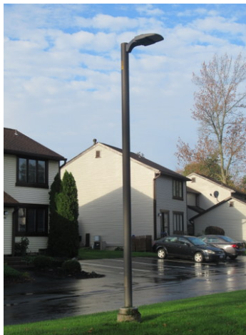
Typical light pole and fixture
