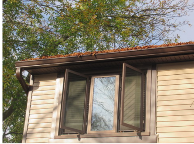
Natural debris buildup and deterioration in gutter of Unit 208
