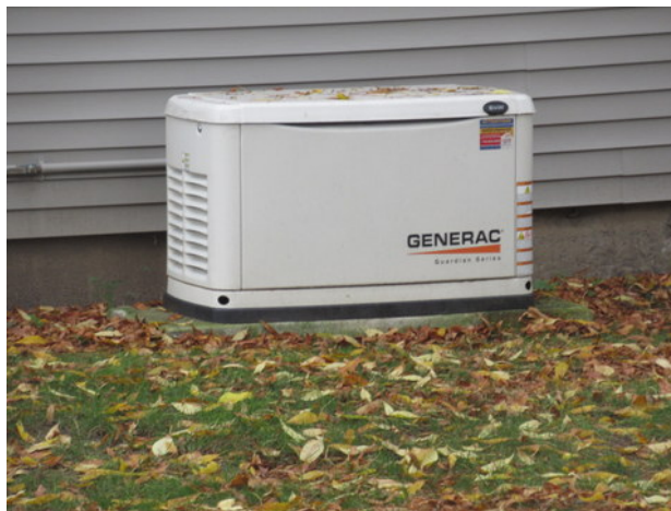
Typical backup generator
