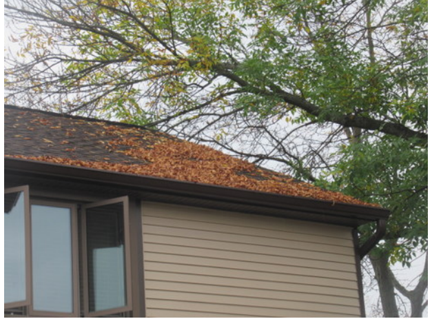
Overhanging and encroaching tree branches, natural debris buildup and deterioration at asphalt shingle roof of Unit 208
