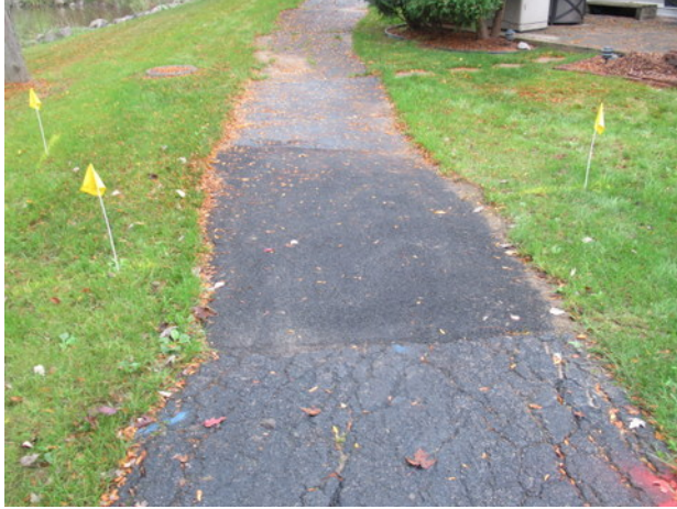
Longitudinal, edge and alligator cracks, previous patch repair and deterioration at asphalt walking path near Unit 1007
