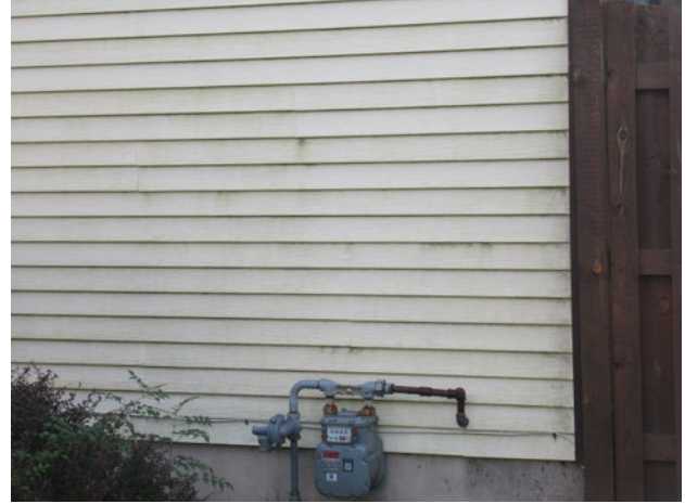
Organic stains and deterioration at vinyl siding of Unit 851
