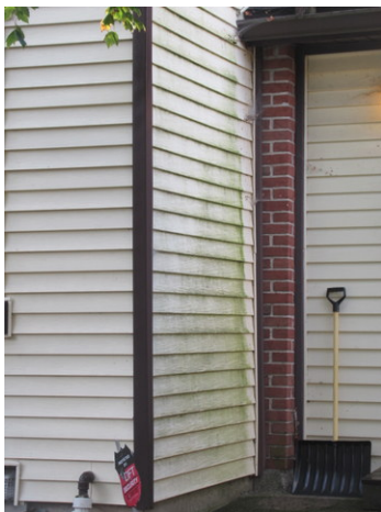
Organic stains and deterioration at vinyl siding of Unit 853
