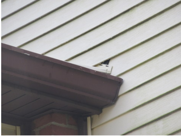
Gap and deterioration at vinyl siding of Unit 851
