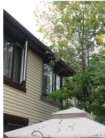
Encroaching tree branches and deterioration at vinyl siding of Unit 354
