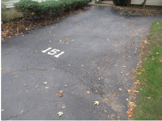
Spider and alligator cracks, and deterioration at asphalt pavement near Unit 151
