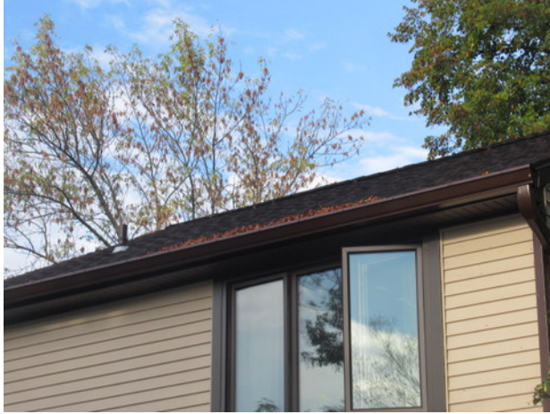
Natural debris buildup and deterioration in gutter of Unit 804
