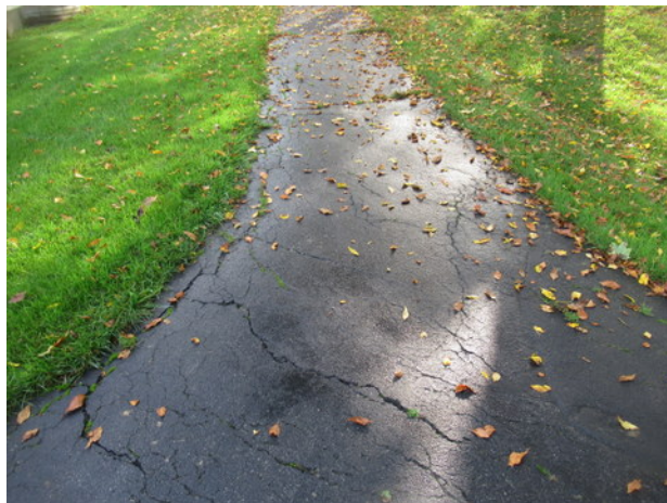
Longitudinal, lateral, edge and alligator cracks, and deterioration at asphalt walking path near Unit 1001
