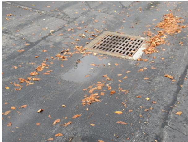
Negative drainage flow, minor settlement and deterioration at catch basin near Unit 1353
