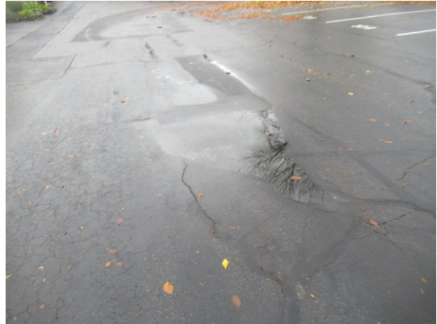
Lateral and longitudinal cracks, previous crack and patch repairs, standing water and deterioration at asphalt pavement near Unit 103
