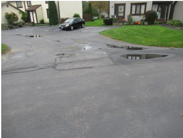
Lateral and longitudinal cracks, previous crack and patch repairs, standing water and deterioration at asphalt pavement near Unit 754
