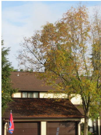
Overhanging and encroaching tree branches, natural debris buildup and deterioration at asphalt shingle roof of Unit 1103
