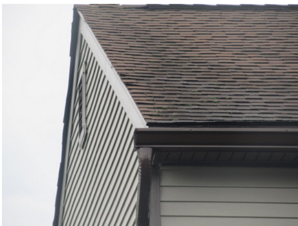
Shingle lift and deterioration at asphalt shingle roof of Unit 754
