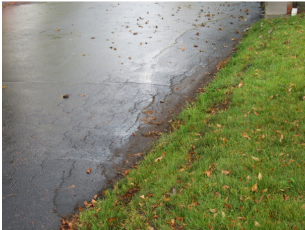
Alligator and edge cracks, and deterioration at asphalt pavement near Unit 1056
