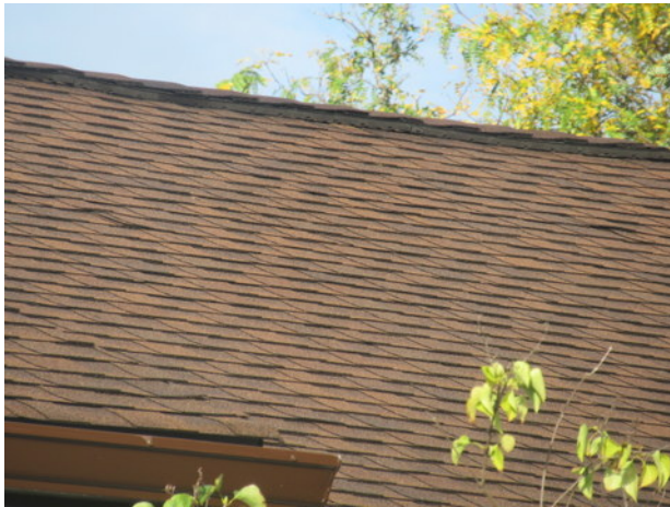
Shingle lift and deterioration at asphalt shingle roof of Unit 502
