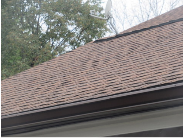
Shingle lift and deterioration at asphalt shingle roof of Unit 1755
