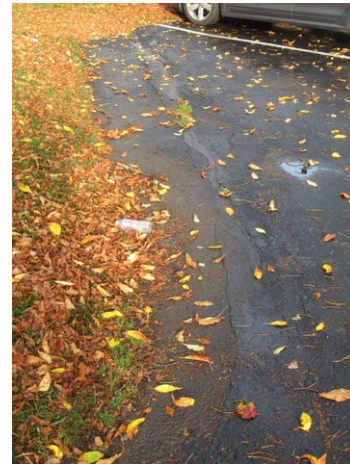
Lateral cracks, standing water and deterioration at asphalt pavement near Unit 804
