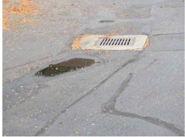
Negative drainage flow, minor settlement and deterioration at catch basin near Unit 1652
