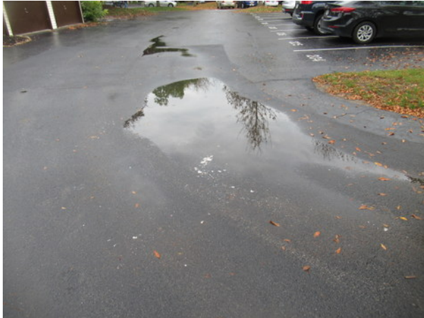
Lateral and longitudinal cracks, previous crack and patch repairs, standing water and deterioration at asphalt pavement near Unit 303
