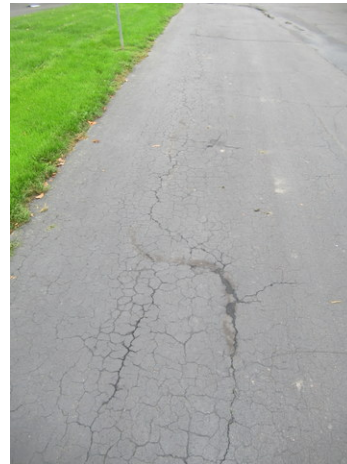
Spider, longitudinal and alligator cracks, and deterioration at asphalt pavement near Unit 851
