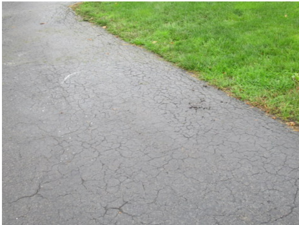
Spider and alligator cracks, and deterioration at asphalt pavement near Unit 353
