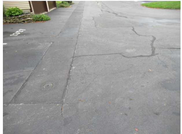
Lateral and longitudinal cracks, previous patch repairs and deterioration at asphalt pavement near Unit 1357
