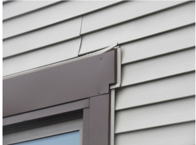
Loose J-channel and deterioration at vinyl siding of Unit 1451
