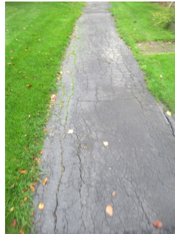
Longitudinal, edge and alligator cracks, organic growth and deterioration at asphalt walking path near Unit 1053
