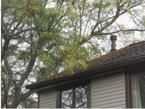
Overhanging and encroaching tree branches, natural debris buildup and deterioration at asphalt shingle roof of Unit 406
