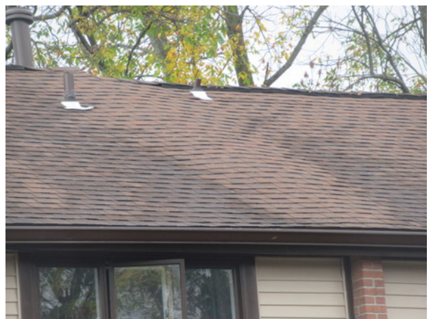
Sheathing deflection and deterioration at asphalt shingle roof of Unit 1353
