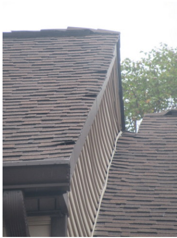
Shingle lift and deterioration at asphalt shingle roof of Unit 203
