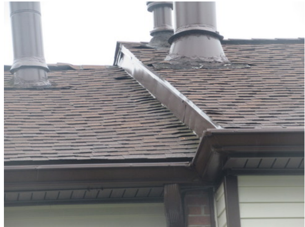
Shingle lift and deterioration at asphalt shingle roof of Unit 1007
