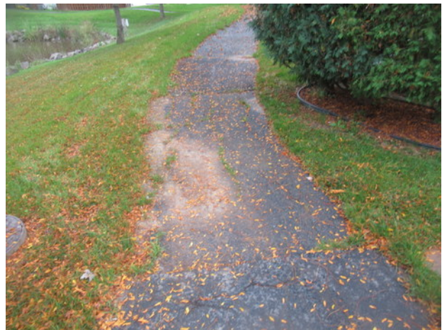
Lateral cracks, previous patch repair, organic growth, minor settlement and deterioration at asphalt walking path near Unit 1008
