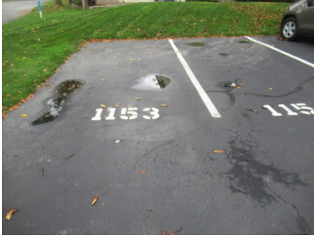
Spider cracks, rutting, standing water and deterioration at asphalt pavement near Unit 1153
