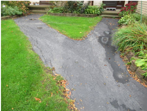
Longitudinal, edge and alligator cracks, standing water and deterioration at asphalt pavement near Unit 1555
