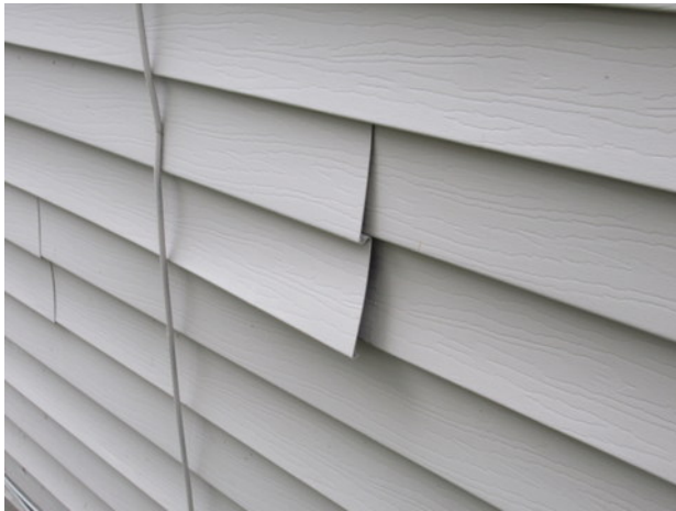
Loose siding and deterioration at vinyl siding of Unit 251
