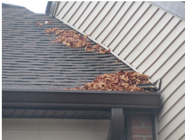
Natural debris buildup and deterioration in gutter of Unit 207
