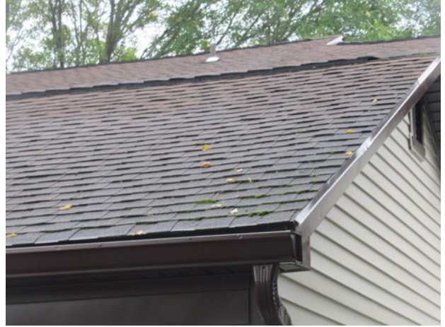
Shingle lift, organic growth and deterioration at asphalt shingle roof of Unit 654
