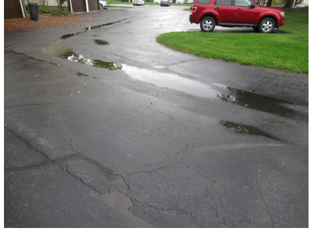
Lateral and longitudinal cracks, previous crack and patch repairs, standing water and deterioration at asphalt pavement near Unit 1102
