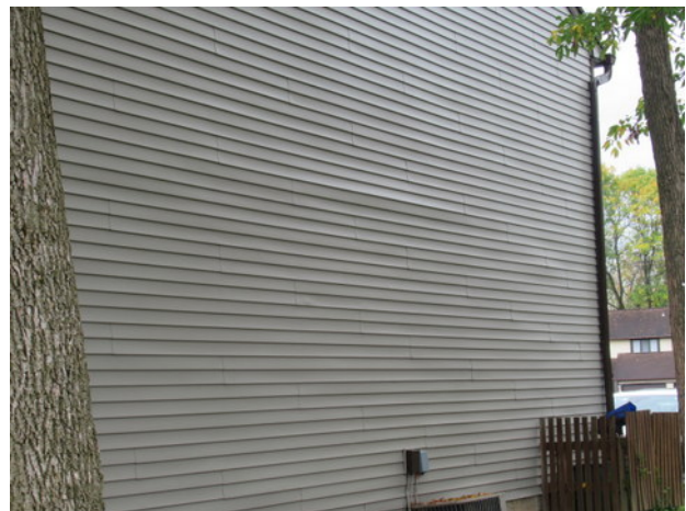
Bulging and deterioration at vinyl siding of Unit 1454
