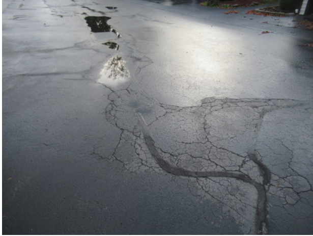
Lateral, longitudinal and alligator cracks, previous crack repairs, standing water and deterioration at asphalt pavement near Unit 1452
