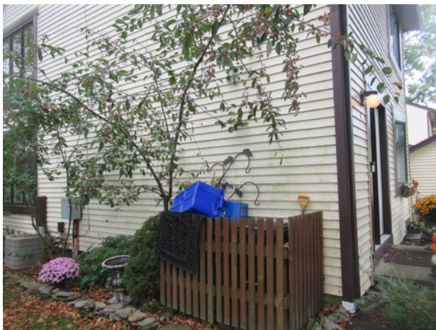
Encroaching tree branches and deterioration at vinyl siding of Unit 1254
