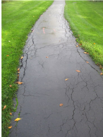
Longitudinal, lateral, edge and alligator cracks, and deterioration at asphalt walking path near Unit 1001
